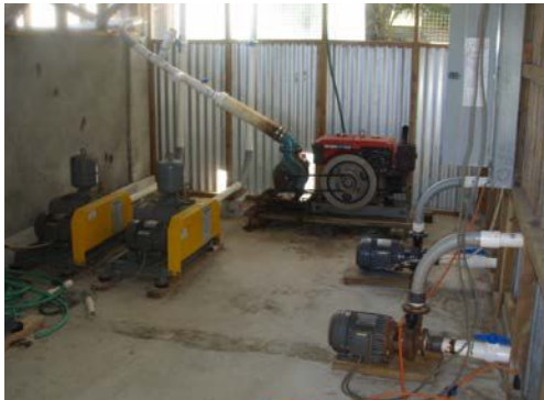
Inside the Pump house
