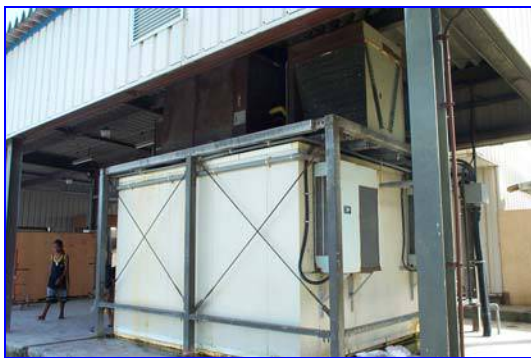
Ice-making machine at MIMRA dock – capable of 5 tons production per day.
